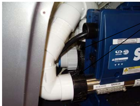
Example of Pump Unions
